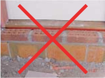
incorrect Kordon TB installation. Refer kd 001 and product design principle
